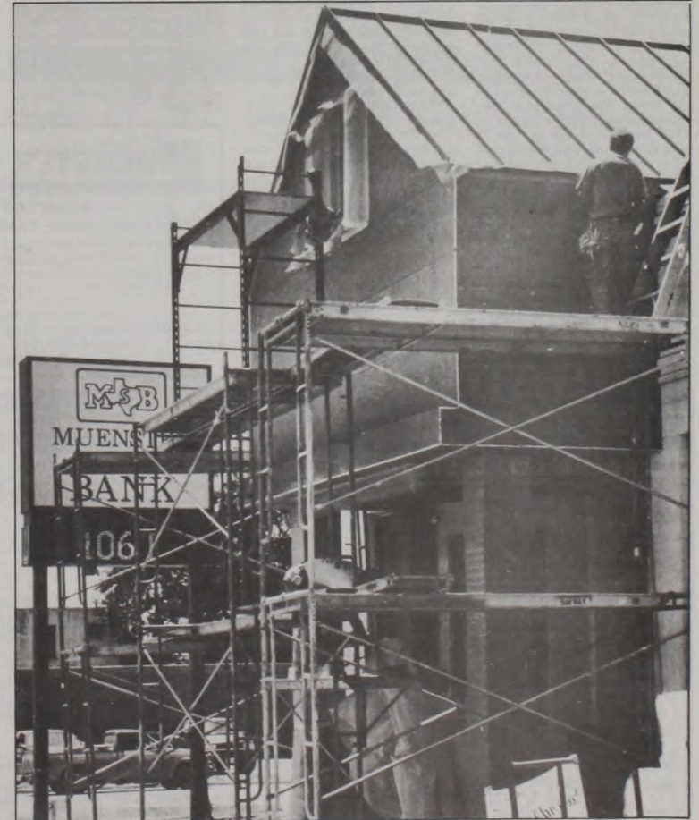
Things continue to rise around Muenster as construction progresses at the Muenster State Bank. The over 100 degree temperatures drag on, with Wednesday being day 18, with little relief in sight. Conditions aren't expected to duplicate the heat wave of '98 which had 42 consecutive 100 degree days. Photo by Janie Hartman
