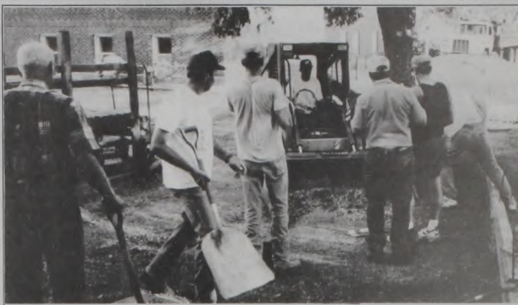
As Sacred Heart School prepares to open, so does the playground. Following some sewer problems, the decision was made to move the manhole rather than move the playground. The area was raised by the level of one landscaping tie and several new layers of gravel were added to the existing layer. Donations are still needed to cover the costs involved and these can be dropped off at the church office and mailed in. Volunteer workers included Raymond Zimmerman, John Bartush, Chris Dangelmayr, Ron Dangelmayr, Ernie Martin, Mike Dangelmayr, and Scott Felderhoff. Courtesy photo
