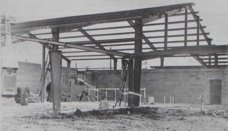
Construction continues on the new Muenster High School building, as the steel framed roof and outer walls begin to give a visible outlook for the new school. Photo by Janie Hartman
