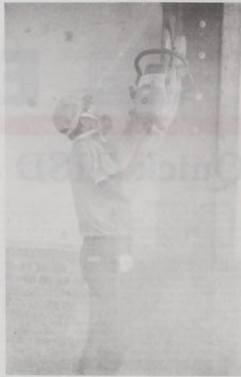
Work continues on the expansion and remodeling at the Muenster State Bank. Workers on Wednesday afternoon began the task of cutting out an opening in the 19 inch wall that separates the present bank from the future expansion. Photo by Janie Hartman
