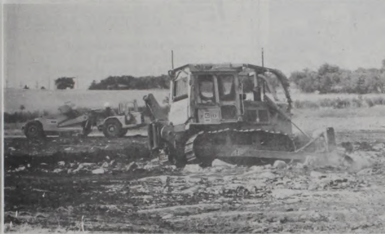
FIELD OF DREAMS - Construction continues at the Muenster Jaycees' future Baseball Complex. Dirt work this week included topsoil on several ball field plots, as the dream of the ball park gets closer to becoming reality. Janie Hartman Photo
