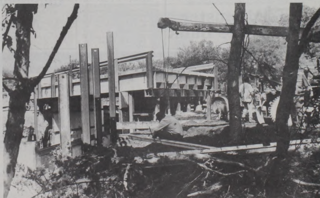
Work continues on a new bridge for County Road 426 northwest of Muenster. Work has been in progress for several weeks to raise the road and install a bridge at a higher elevation. This is necessitated by the potential flooding to the present road when Lake Muenster is built.
