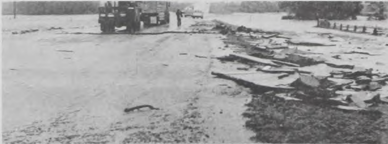
The ravages of Tuesday's flood caused this pavement damage on Highway 82 between Myra and Lindsay. Janie Hartman Photo
