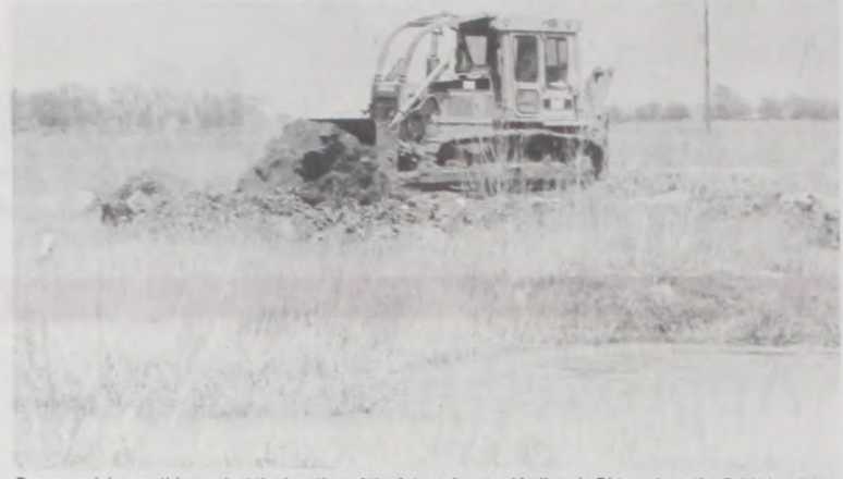
Dozer work began this week at the location of the future Jaycees' ball park. Dirt work on the fields has been postponed time and time again due to rain. The Muenster Jaycees began the Little League Baseball Program in 1963 and hope to keep the tradition going stronger than ever with the new ballpark complex. Janie Hartman Photo
