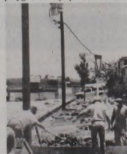
Repairs to the Muenster ISD Elementary building continue, including a new roof cover being installed by Structures, Inc., and new curbing by Barnhill Concrete. Janie Hartman Photo
