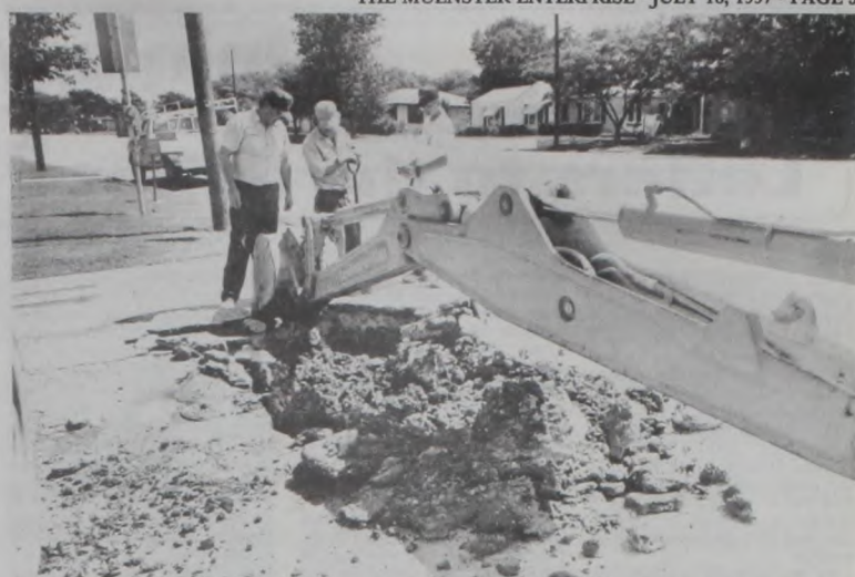
A water leak was discovered on West Eighth Street near Main last week and quickly repaired by city workers, Chris Yosten, David Dittfurth and Royce Knabe, with Fleitman Backhoe digging the hole. Janie Hartman Photo
