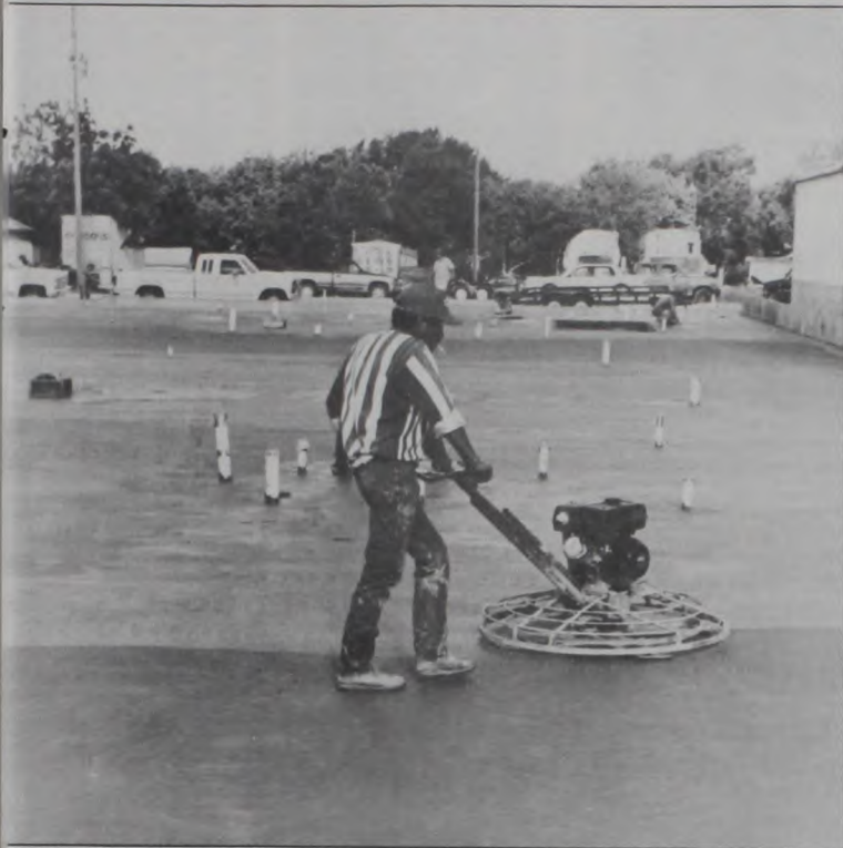
CREW OF MORE THAN 30 began work very early Wednesday morning in pouring the concrete foundation for Fischer's Meat Market. The expansion of the store is now in full swing after Butch and John Fisher removed the unstable Wolf building in February, 1995.
