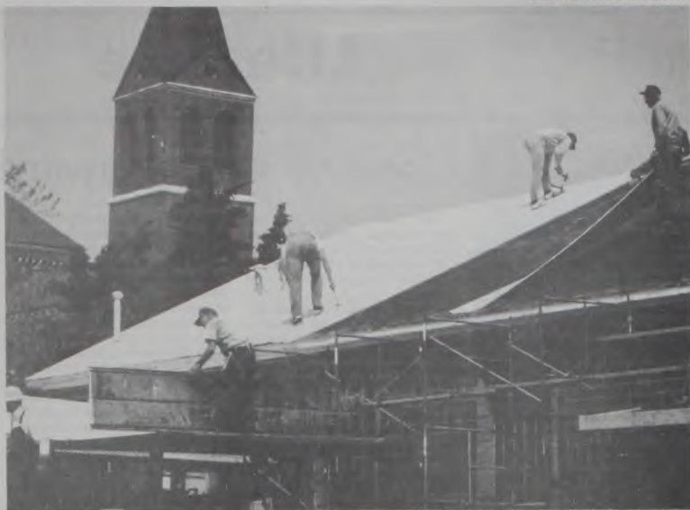
Norb Mages helps Lindsay KC Grand Knight Gene Pelzel remove old roofing material from the Parish Hall. The KCs replaced the 50 year old roof with new metal. The appearance of the new roof matches the church and surrounding buildings. It was the result of many volunteers and donations and was also the first major project for the new Lindsay KC Chapter.
