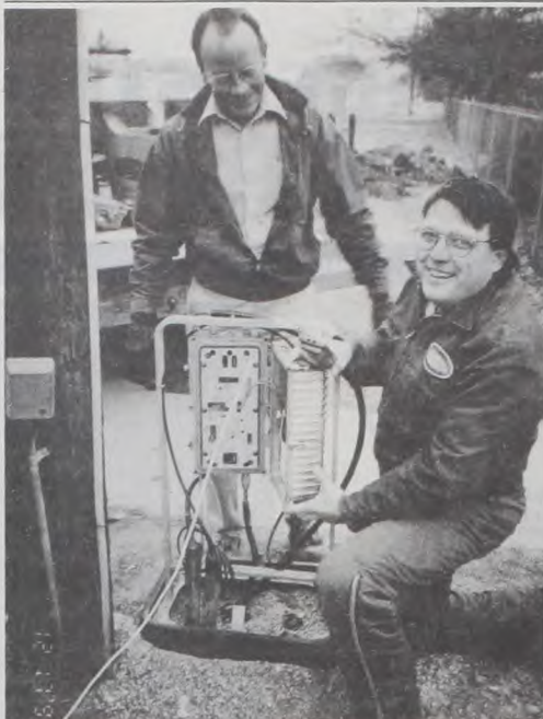
Joe Yosten, kneeling, shows Lindsay Mayor Robert Walterscheid the Lindsay Fiber Optic Connection to the Muenster CATV system. Courtesy photo
