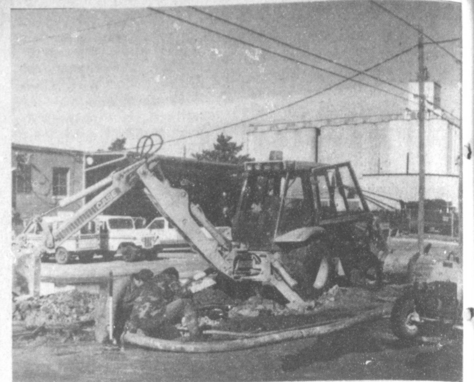
A SCENE REPEATED ALL OVER MULESHOE--For about a week, workers from the City Water Department have been busy day and night replacing burst water mains, such as the one shown here just east of the post office. They also had frozen and burst water meters, and many instances of burst pipes, with people calling in needing their water turned off "real fast." Another cold front was approaching the area late Friday afternoon, with freezing rain and snow predicted for the weekend. (Journal Photo)
