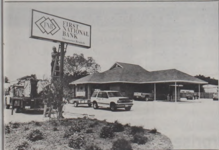
John Schneider's sign company of Denton installs the new sign for First National Bank, Muenster Branch, which opened Wednesday morning on Highway 82. Photo by Janie Hartman
