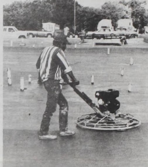
A crew of more than 30 worked at pouring the foundation for Fischer's Meat Market. Janie Hartman photo
