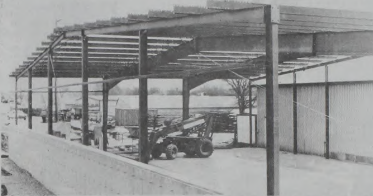
Construction at Flusche Enterprise, Inc. in Muenster. The expansion of the business includes a 60'X100' enlarged work area and a 30 square foot office. Staff photo
