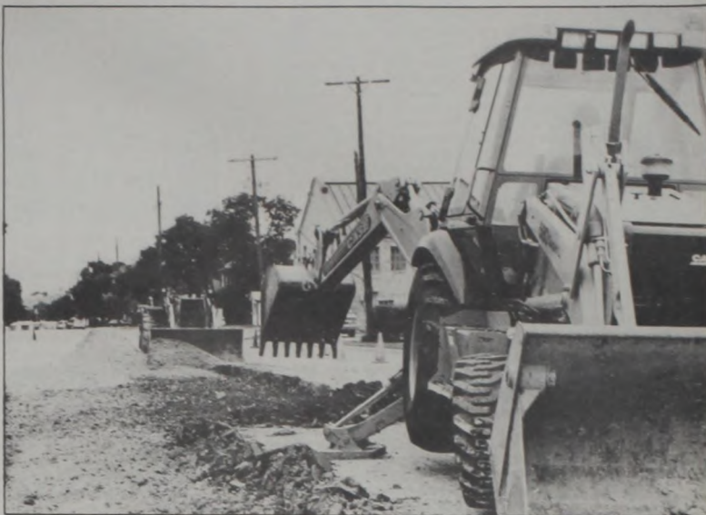
CITY WORKERS have been busy this week preparing damaged streets in Muenster. The work includes removing the crumbling pavement and several inches of gravel, dirt and clay, then filling the area with filler rock and dirt that will be packed in preparation for a new pavement. Workers are pictured Wednesday afternoon on Oak Street.
