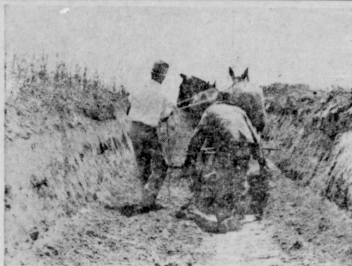
Trench silos of the type shown above have proved useful in Brown County for winter feeding purposes during the past few seasons. The above is a 140 ton trench silo under construction. It was filled with grain sorghum which was used as roughage in feeding stock for the market.
