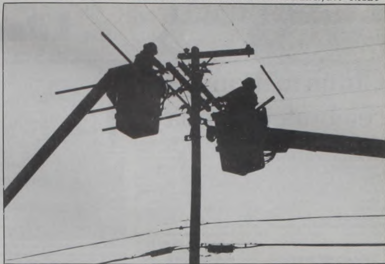
TU ELECTRIC technicians are silhouetted against the evening sky Monday as they worked to reroute power lines and repair a broken cross-arm. Dave Fette Photo
