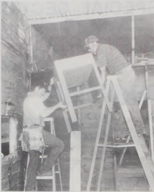
BRIAN COUGHENOUR , left, and Roland Bell bring down one of several "treasures" found in the remodeling of the old Floyd's Bar on Main Street. Removal of charred boards from the wall "behind the bar" opened an area closed for many years. Rick and Sydney Reynolds are restoring the building for a new business venture in Muenster. Janie Hartman Photo
