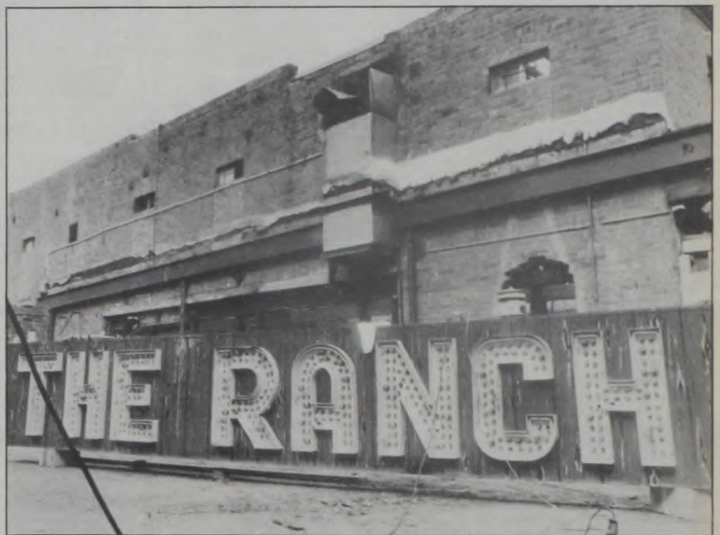
A MUENSTER LANDMARK, known to the younger generation as "The Ranch," will soon be leveled for the expansion of Fischer's Meat Market. Original plans to restore the building were changed when it was discovered the building was unstable. Historically known as the Wolf Building, the structure was built in 1927. Janie Hartman Photo
