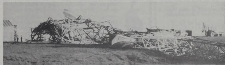
AT&T's MICROWAVE TOWER near Forestburg was mangled and blown down Sunday. Montague residents lost their outgoing long distance service. At right, workers construct a new tower on the site. They worked quickly and had made this much progress by Monday evening.
