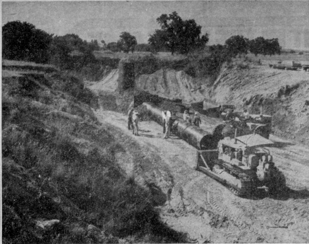
THE BULCHER SPECIAL ACP Project which was approved for the northwest corner of Cooke County in 1970 has been very successful. Seven grade stabilization structures were built and 76 acres of gullies have been shaped and established to bermuda grass. Interest in the project was very good the first year. Landowners have done an excellent job of carrying out a program which not only helps keep their land in place but stops silt from entering Moss Lake and Red River. These areas will need careful management to keep a cover of grass on the shaped area. The project has been approved for 1971.
