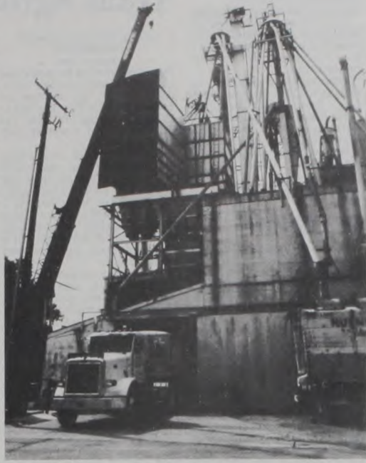
WORK CONTINUES at Muenster Milling's North Main Elevator, including the placement of a second new ingredient bin. The bin was constructed at the site, then lifted 67 feet by a crane to its new location.
