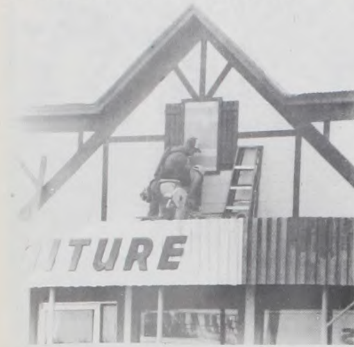
CHANGES on the exterior of Hess Furniture Company, to lend ethnic decor, are constructed by Rudy Koesler and one of his helpers.
