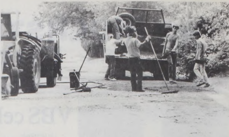
CITY WORKERS continue repairing the many washed and worn streets in Muenster. The repairs are being done with the assistance of workers hired for the summer.
