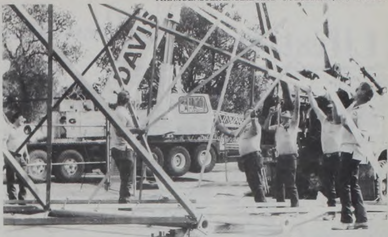
EMPLOYEES of Muenster Telephone Company dismantle a section of "the tower." Workers include, l to r, Joe Yosten, Maurus Hacker, Larry Eldridge, Donnie Hellman, Robert Williams and John Monday.
