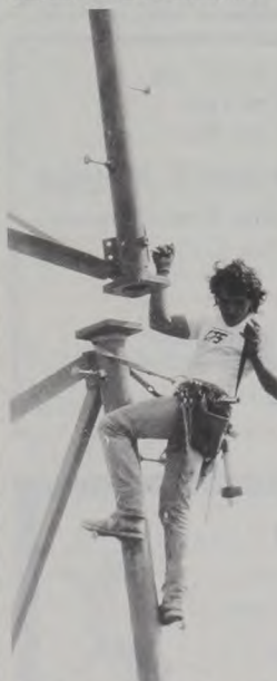
A WORKER from Lumberton Tower Service places his tool in his belt as another section of the tower is lifted, to be dismantled earlier this week. Janie Hartman Photo
