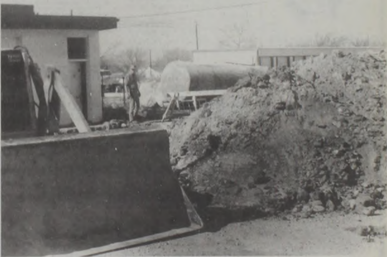
Speedy Reiter looks at the large hole next to his service station where fule tanks were once buried. Strict, expensive government inspection of commercial underground storage tanks is causing many small gas stations to close down. Tanks are subject to be registered by the Texas Water Board and tested every year, at the owner's expense, for leakage. Tanks not used in 15 years are not required for inspection. Speedy said he's still undecided about his future plans. Janie Hartman photo
