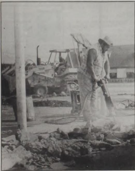
Workers from North Texas Pump Company of Denton demolish the pump island at Speedy Reiter's gas station early this week. Herr Oil Company of Gainesville recently abandoned the location, removing the underground gas tanks. The Texas Water Commission then ordered all lines removed. Similar work was done at Dude Grewing's station to repair ventilation lines. No gasoline leaks were found at either location, but Dude's cannot pass inspection until the lines are repaired. Janie Hartman photo
