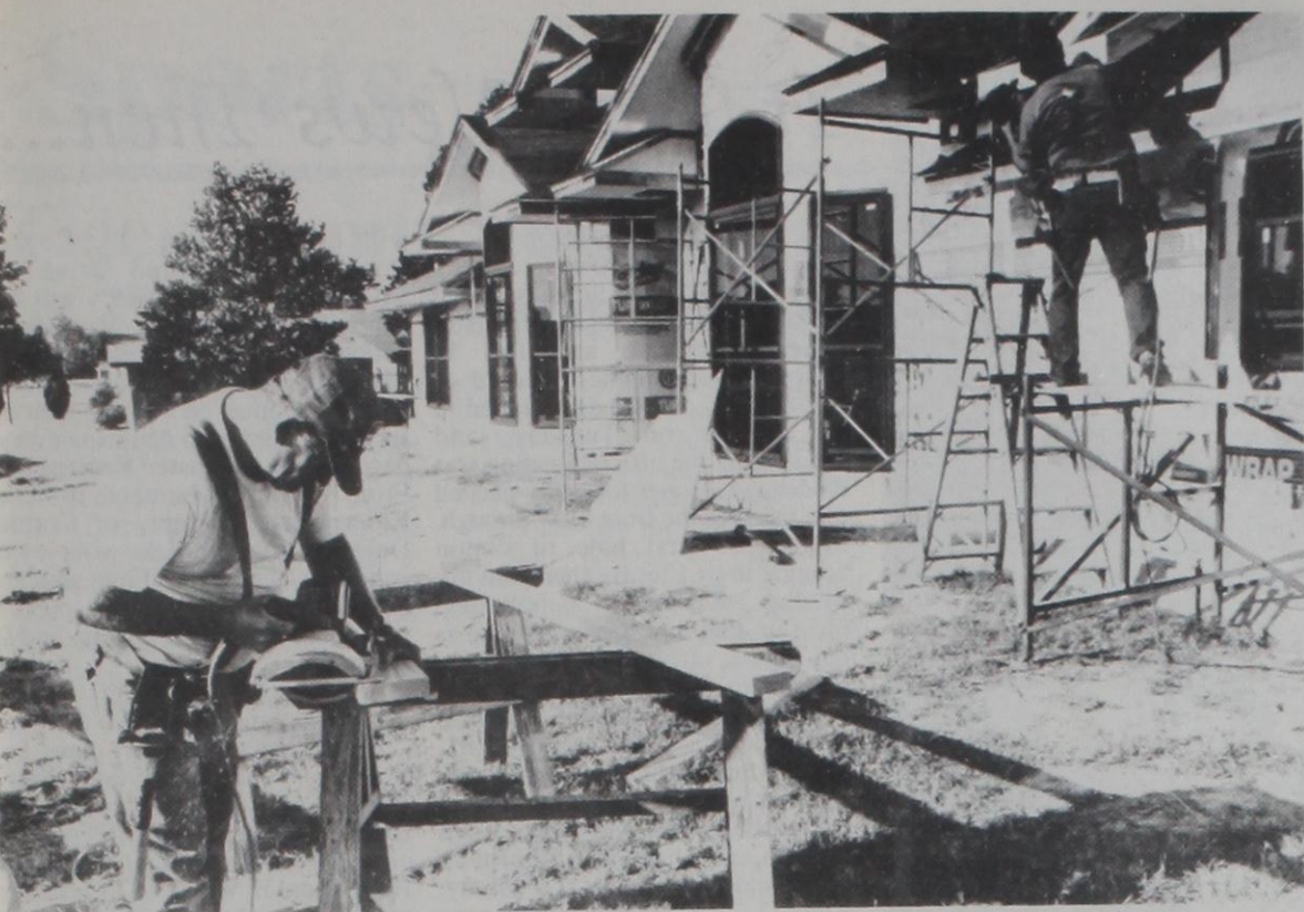
DAVID VOGEL, left, and Steve Yosten are constructing a new home on Elm Street for the Terry Rohmer family. Construction of new homes has picked up in recent months for the Muenster area. Watch next week's Muenster Enterprise for a story on building. Janie Hartman Photo
