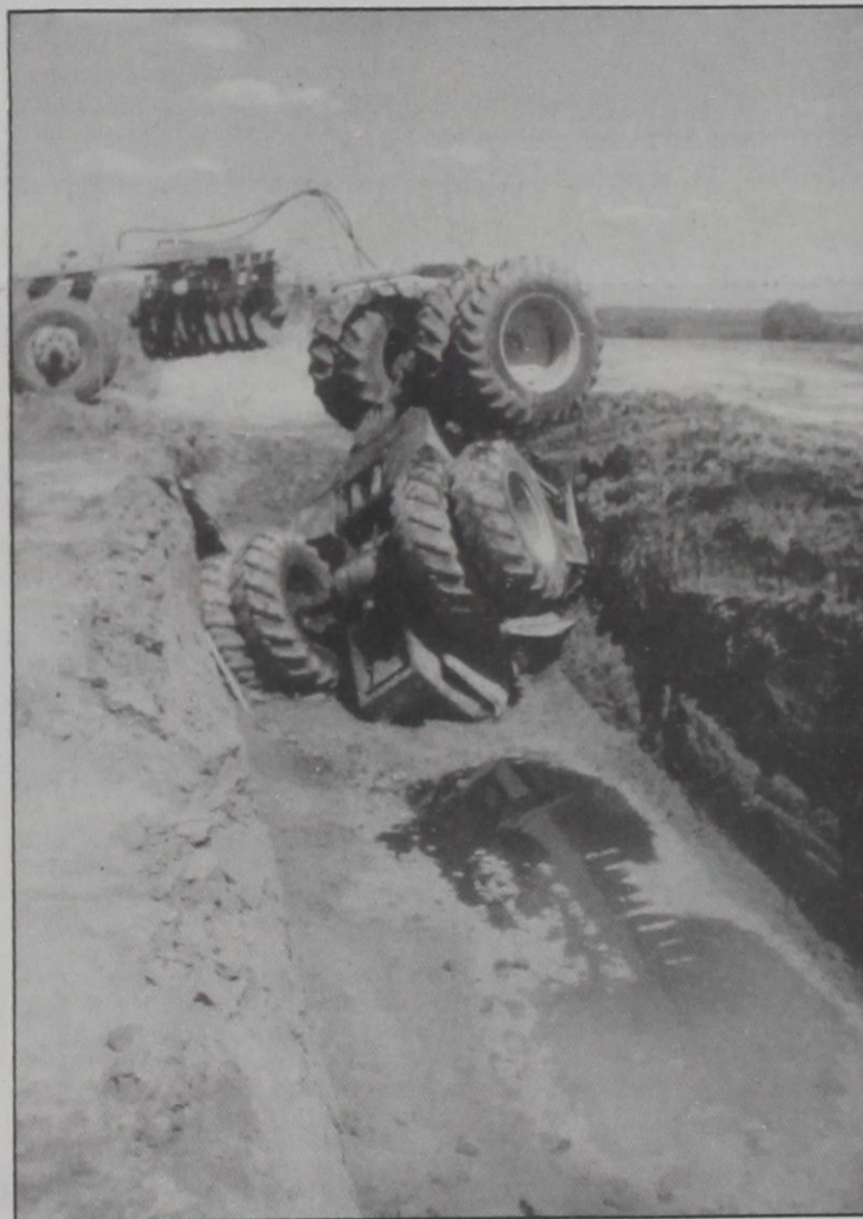
JEFFREY SEWELL was killed after being pinned under this large John Deere tractor last Friday at the construction site of the new Red River Bridge. Courtesy Photo
