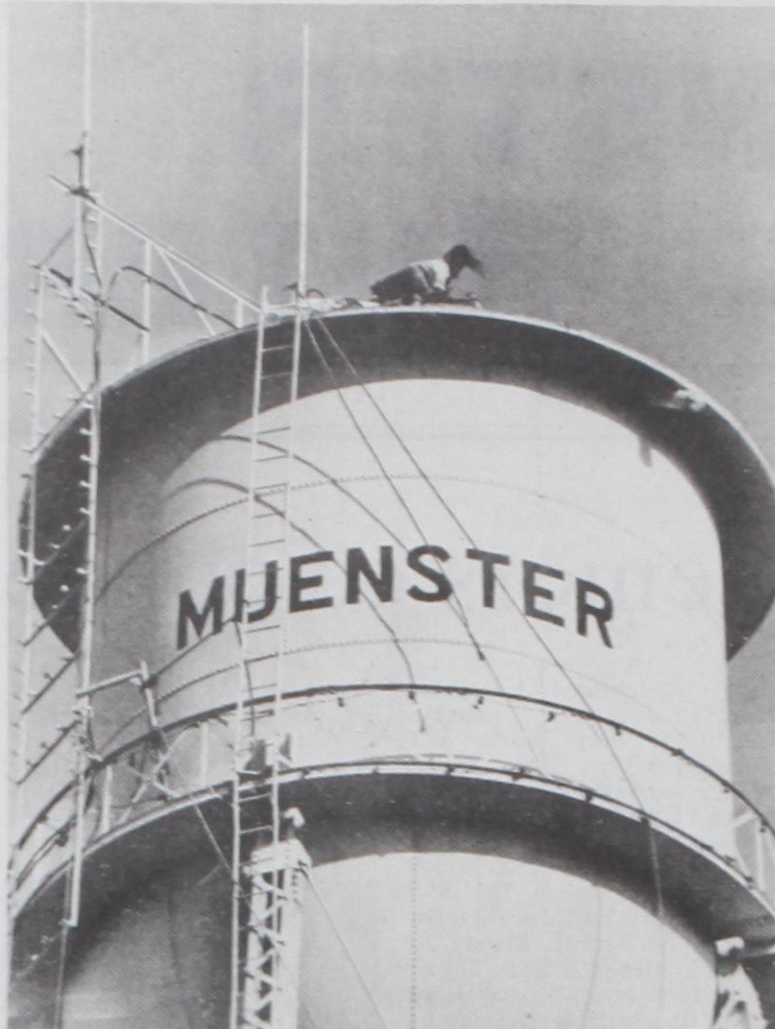
WATER TANK MAINTENANCE of Grove, Oklahoma began work on Muenster's water tower last week Friday. After sandblasting the interior of the tank, welding 12 holes shut and repairing the rusted stand pipe, the crew finished fiberglassing the inside Wednesday. It should be another week before the tank can be filled, to allow the finished work to dry. Janie Hartman Photo
