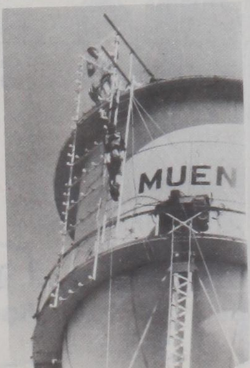
Radio tower mounted on water tower.
