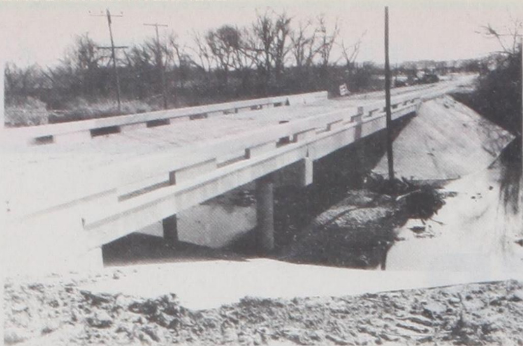
THE NEWLY-INSTALLED BRIDGE over the Brushy Elm Creek is near completion. Construction was started in late September.
