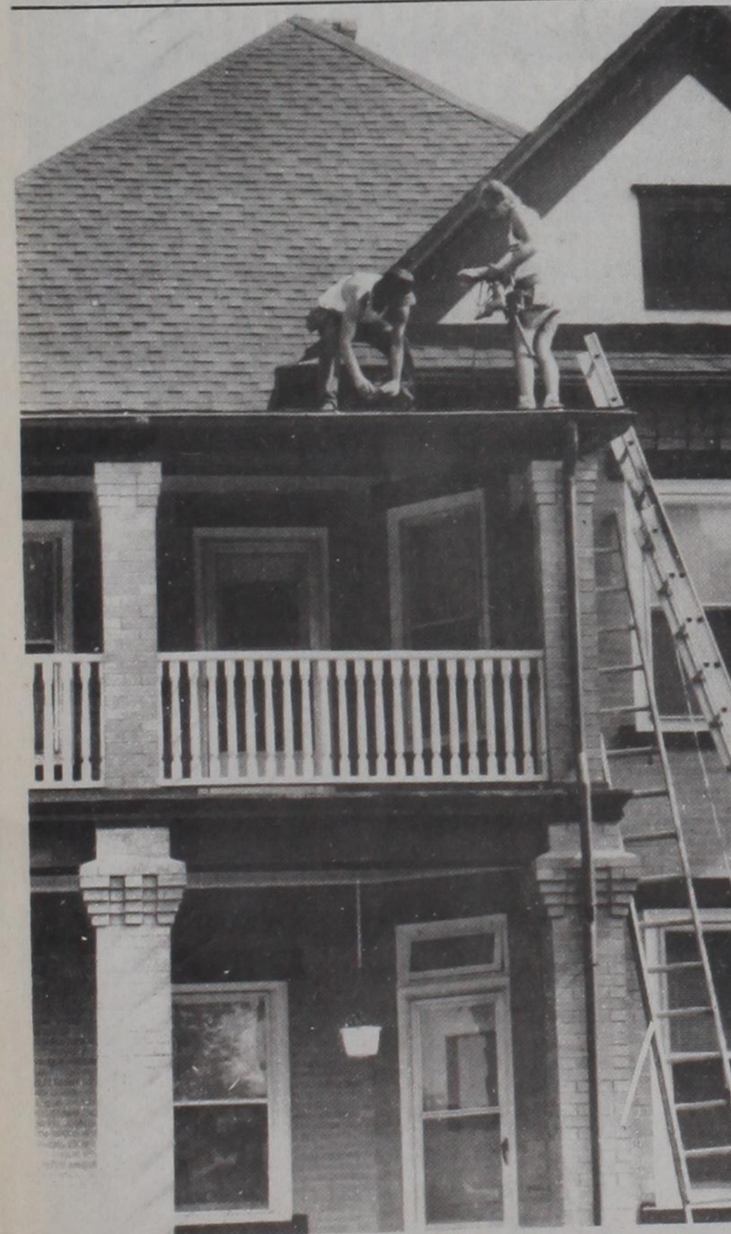
ROY WILLIAMS and Dee Bell of Gary Bell Construction of Forestburg replace the drain pipes on the Sacred Heart rectory recently as part of the outside fix-up on the parish grounds. Other improvements were the painting of trim on the rectory and convent and painting the meeting room in the Community Center. Janie Hartman Photo
