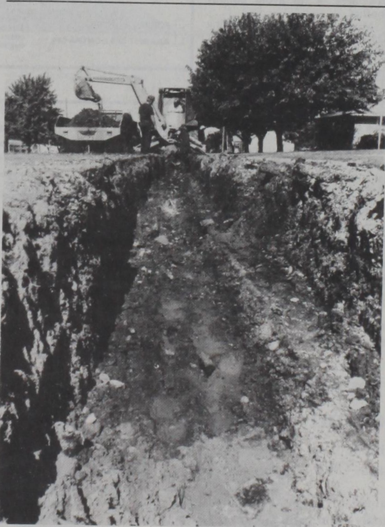
CITY OF MUENSTER employees, l to r, Joe Fenton, David Dittfurth, and Tony Hess and Bernard Hesse of G&H Backhoe dig a trench in preparation of replacing 280 feet of cast iron water line with PVC pipe. The work is being done along Sixth Street. Leaks have required repairs several times during recent years. These were done with patch clamping. The weakened base has caused street damage and the new pipe should eliminate the problems. Janie Hartman Photo
