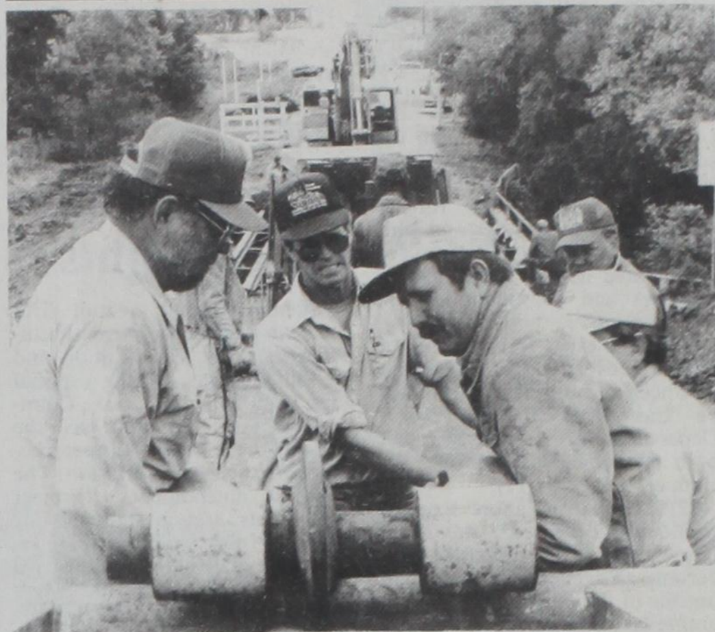
THE OLD ASH STREET bridge over the Brushy Elm Creek was removed Friday to make way for a new one. The picture at left shows Cooke County Precinct 4 employees Wayne Trubench (left) and Billy Poyner (right) working with Tim Hess (center) and Herkey and Jim Biffle of Gainesville Trucking Co. setting the poles and cable which will lift the bridge out of place. 4 Commissioner Virgil Hess said the estimated 30,000-pound bridge will be used to replace a condemned span northwest of Muenster near Dave Flusche Sr.'s place.
