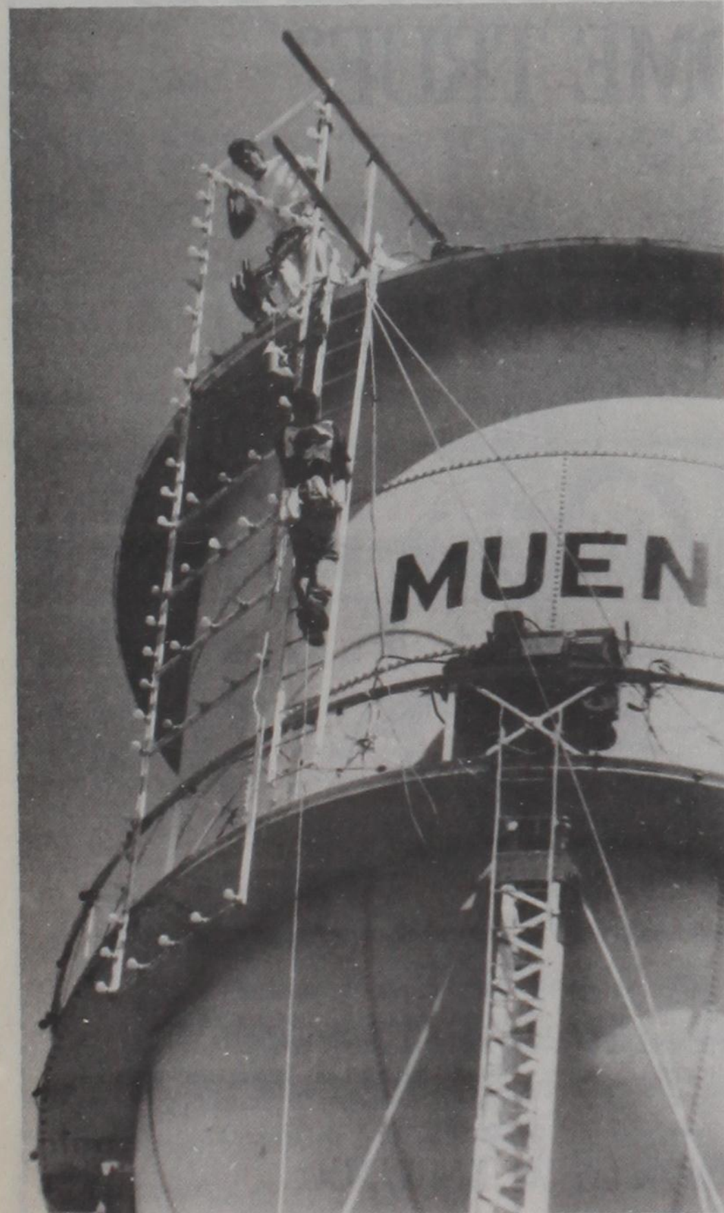
JERRY MURLEY, top of tower, and Ronny Livingston, on ladder, assisted by Tommy Prosize (not shown) work to install a cellular telephone enhancer on the Muenster water tower. The men are employees of EL-COM and Associates, Inc. of Plano. The company has been contracted by Southwestern Bell Mobile Systems to install the tower. The antenna is 1150 feet above sea level (150 feet off the ground) and will pick up cellular phone signals in this area and re-transmit them to the Gainesville tower. The system should be operational this week and will greatly improve cellular phone service in Muenster as well as north and west of Muenster. Southwestern Bell Mobile Systems is renting the space from the city. Janie Hartman Photo
