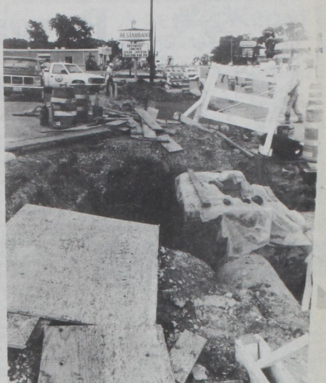
JOHN BARTON, engineering assistant with the Texas Highway Dept., reports that construction to install storm sewer pipes along Hwy. 82 in Muenster is progressing as expected. Estimated time of completion is three weeks. Driveway, curb and gutter work is lacking on one side of the highway and three inlets must be installed. The work is being done to alleviate street flooding during heavy rains. "So far, it seems to carry the flow and seems like it will function well," said Barton. "But the true tests will come when the inlets are completed." The construction work was contracted by Bay Maintenance Company, Inc. of Horseshoe Bay. Work began on April 2 and is being done between FM 373 and the intersection of Pecan Street and US 82.
