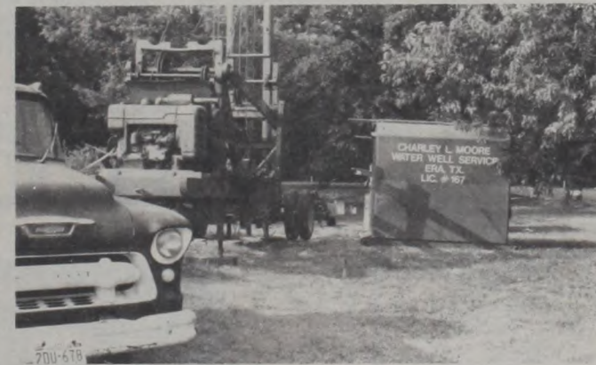
The latest contribution to Muenster's appearance is now in process as the Jaycees provide a water well for watering lawns and shrubbery at the city park. It is located west of the swimming pool. The entire installation, including drilling, pipe and pump, is being paid for by the Jaycees. Staff Photo
