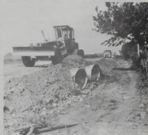
EMPLOYEES of Cooke County Precinct 4 level out County Road 426 north of Muenster after replacing the small tin horns with two larger ones and raising the road 4 to 5 feet. The road had been flooding badly. The bar ditches are also being cleaned out and the excess dirt used as fill to raise the road. County Commissioner Rosalee Bayer said the crew has recently finished extending the bridge at Black Hollow (near Marysville) 40 feet because of wash out. They have one more bridge damaged by heavy spring floods to repair. Janie Hartman Photo
