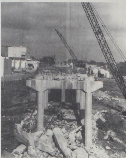
After slightly more than a day, the 41 year old Muenster overpass was reduced to this condition by two 8000 pound wrecking balls. It is being replaced by a four lane surface road.
