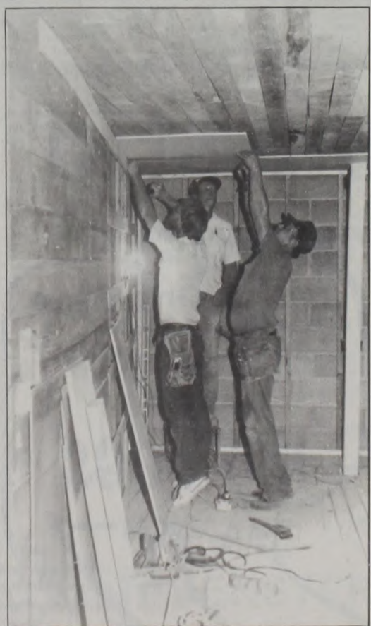
WORKERS continue remodeling in the Old Theatre Mall, in preparation for two new businesses to be opening soon - a jewelry store and a shoe store. Pictured above, Fred Koesler, Dale Klement and Waylen Poole work in the old "projection room," upstairs of the mall where the shoe store will be located. Janie Hartman Photo
