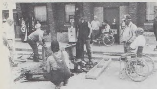
VALLEY VIEW CITIZENS got together this past week to construct the first handicapped ramps on the square in the town's history. All the materials and labor were donated for the job, which placed ramps on the east and south sides of the square. Handicapped parking and handicap access signs are expected to arrive this week.
