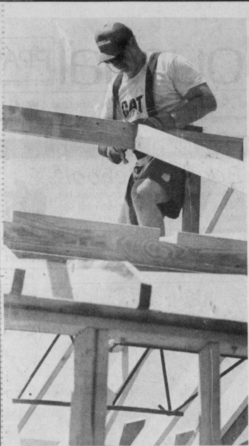
HARD AT WORK — David McIntire, pastor of New Vision Church of the Nazarene, works on a 3,200 square foot addition being added to the church. The church has received a great deal of support from community volunteers.
