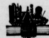
A mechanical cleaning machine brushes dust from the outside of the pipe line, then applies a coat of primer.
