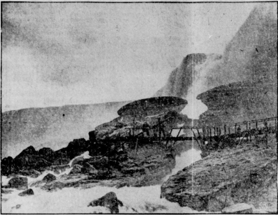
Under the brink of roaring Niagara where a misstep may mean death, workmen in oilskins are seen erecting the wooden footbridge across which 1935's honeymooners and sightseers will scamper to marvel at the Cave of the Winds and Niagara's terrifying might. Because of mild weather, the bridge-builders have undertaken their annual task on the slippery rocks at the earliest date within memory.
