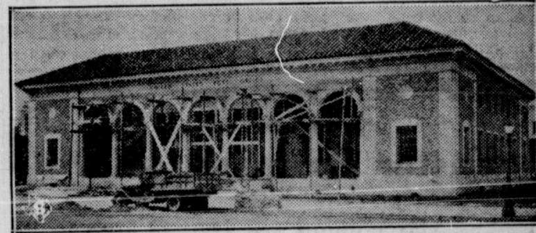
The new postoffice building for Plainview is being completed in record time and is expected to be ready for occupancy about April 15. It cost $125,000.00.
