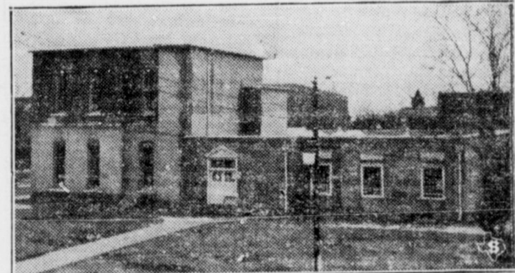
Around the blackened skeleton of the old Grayson county court house, burned in 1930 at the height of the trial of a negro for attacking a white woman, this temporary structure, now nearing completion, is being built to house the county offices at Sherman, Texas. The story part of the building utilizes the only part of the old courthouse that wouldn't burn—the vault in which the negro was cooked to death.
