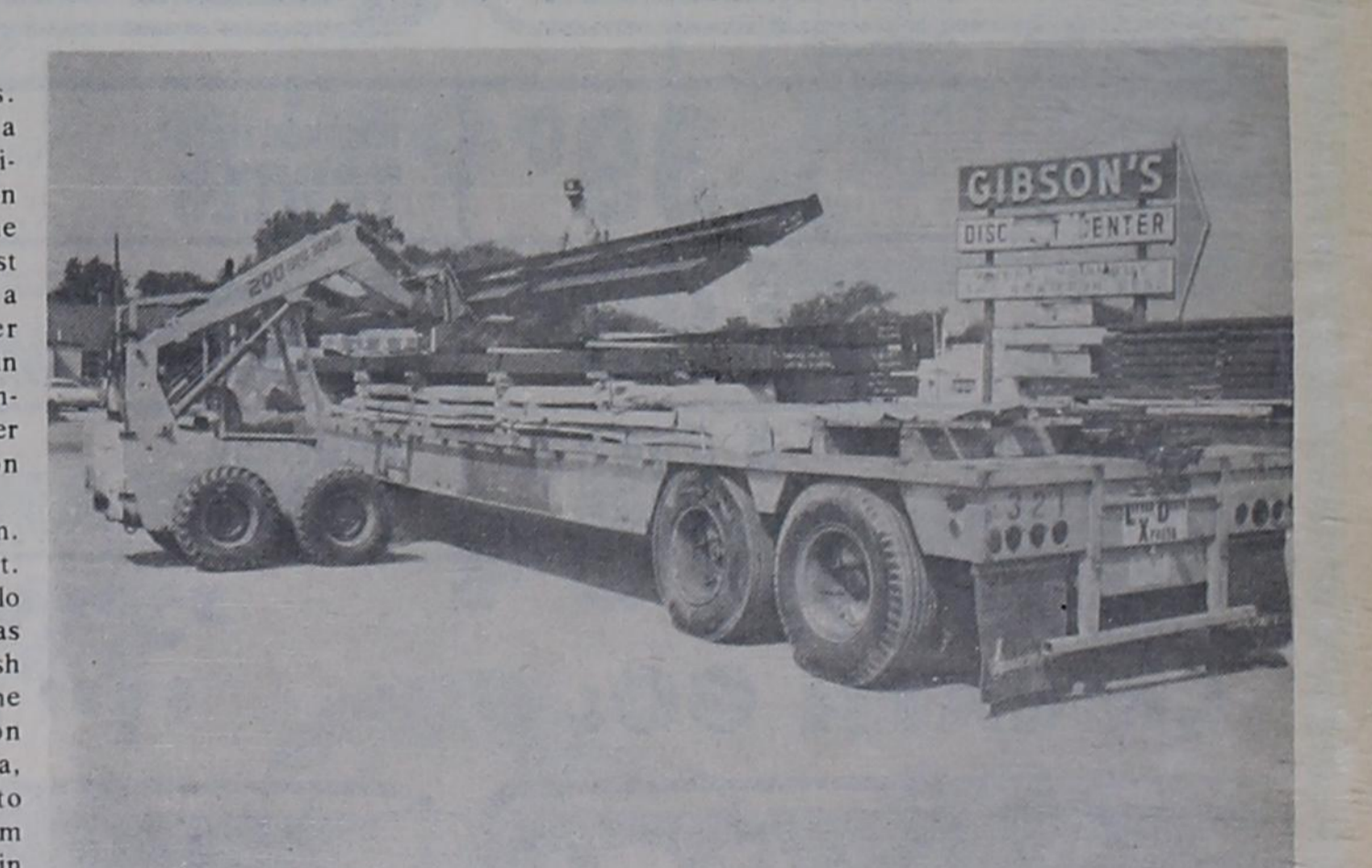
HALLMARK BUILDERS contractors for Gibson's new building have something to work with as the arrival of this load of steel shows. Work is near completion on the slab
