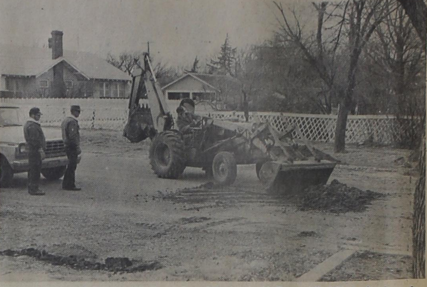
CITY MAINTENANCE PERSONNEL [l to r] Craig Pillard, Jake Moffett and Park Taylor finish another mending job on storm damaged water pipe.
